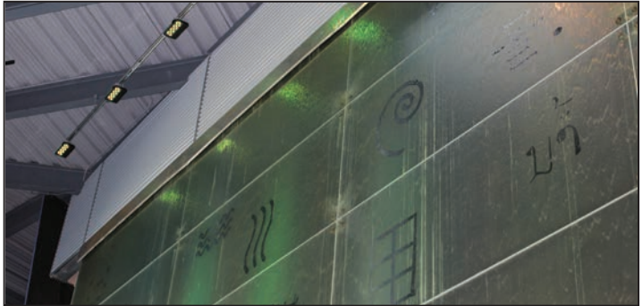
LED lights on the water wall in the lobby of the Great Lakes Aquarium demonstrate energy savings and versatility.
