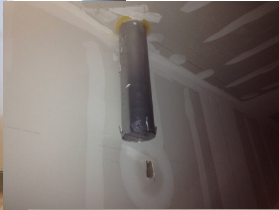
Exhaust fan ducts
