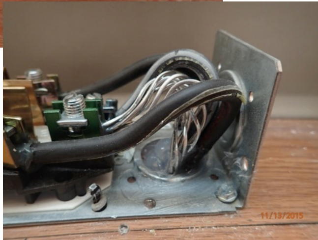
Range electric line
