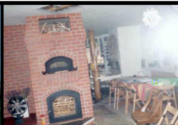
Fig. 2: Masonry Heater in living room
