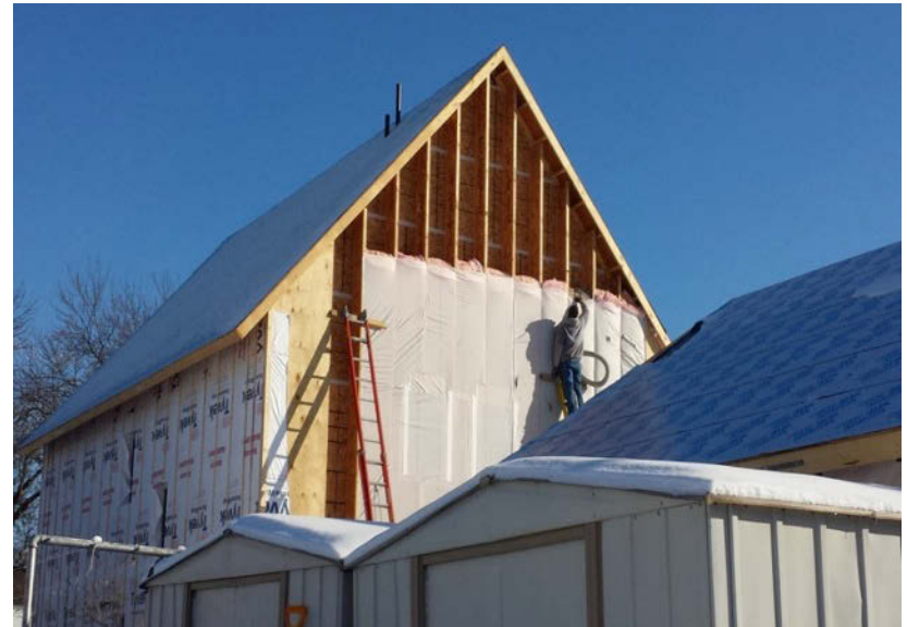
Dense Pack Cellulose, fiberboard and Tyvek (note the furring strips for air gap)
