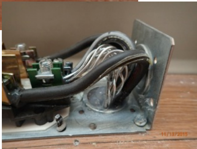
Range electric line
