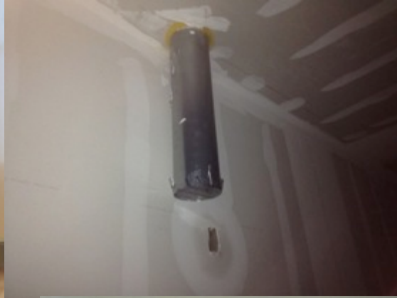
Exhaust fan ducts
