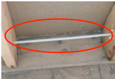
Bottom plate/sheathing gap
