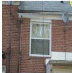
Defective gutters = water leaks
