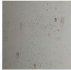
Water leaks = mold hazards
