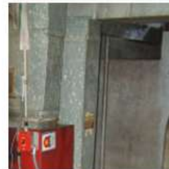
Broken ducts = higher heating bills
