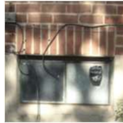
Deteriorated windows = air leaks
