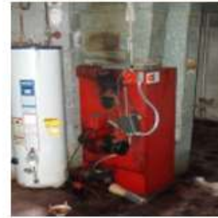
Broken hot water heater and furnace
