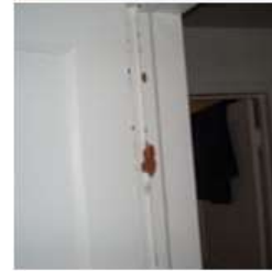
Chipping paint = lead hazard
