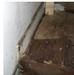
Broken tile = safety hazard
