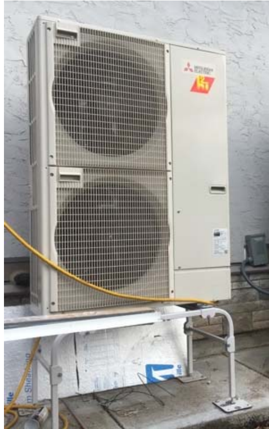
Ducted Whole-House Installation, All-Electric
