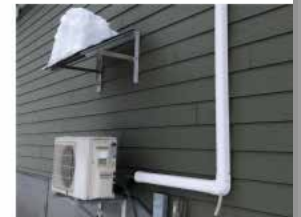
Proper outdoor placement, showcasing a drip cap/snow shield.
