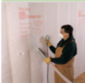
No gaps or voids
