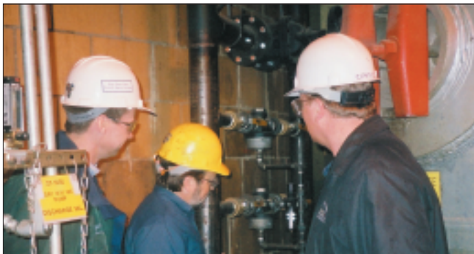
Minnesota Power Energy Consultant Matt Haley, GP Superintendent of Maintenance & Engineering Dale Reed and Clayhill® Sales Engineer Bill Mestelle inspect the new control valve on GP's compressed air distribution system.
