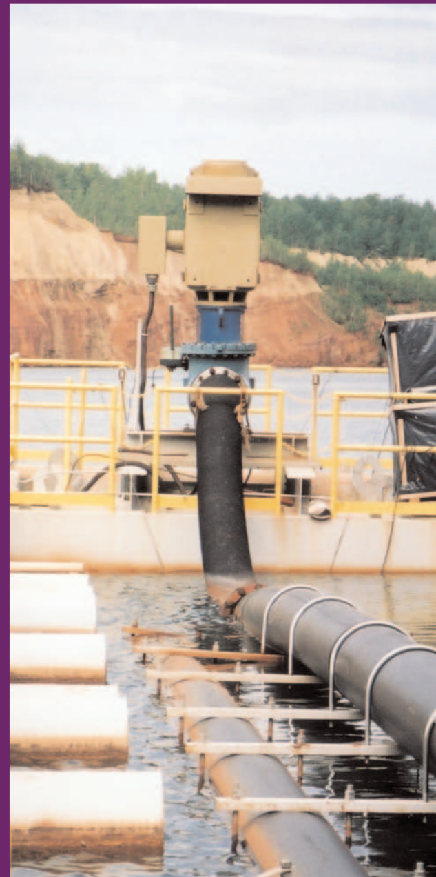
The new electric pump at Hill Annex Mine saves the State of Minnesota more than $100,000 per year.
