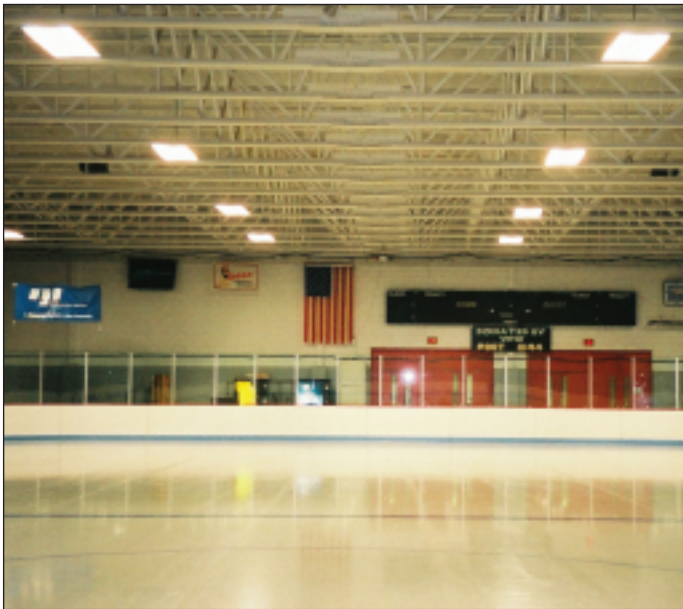
High-bay fluorescent lighting over the rink will save the City of Hoyt Lakes $3,900 per year.
