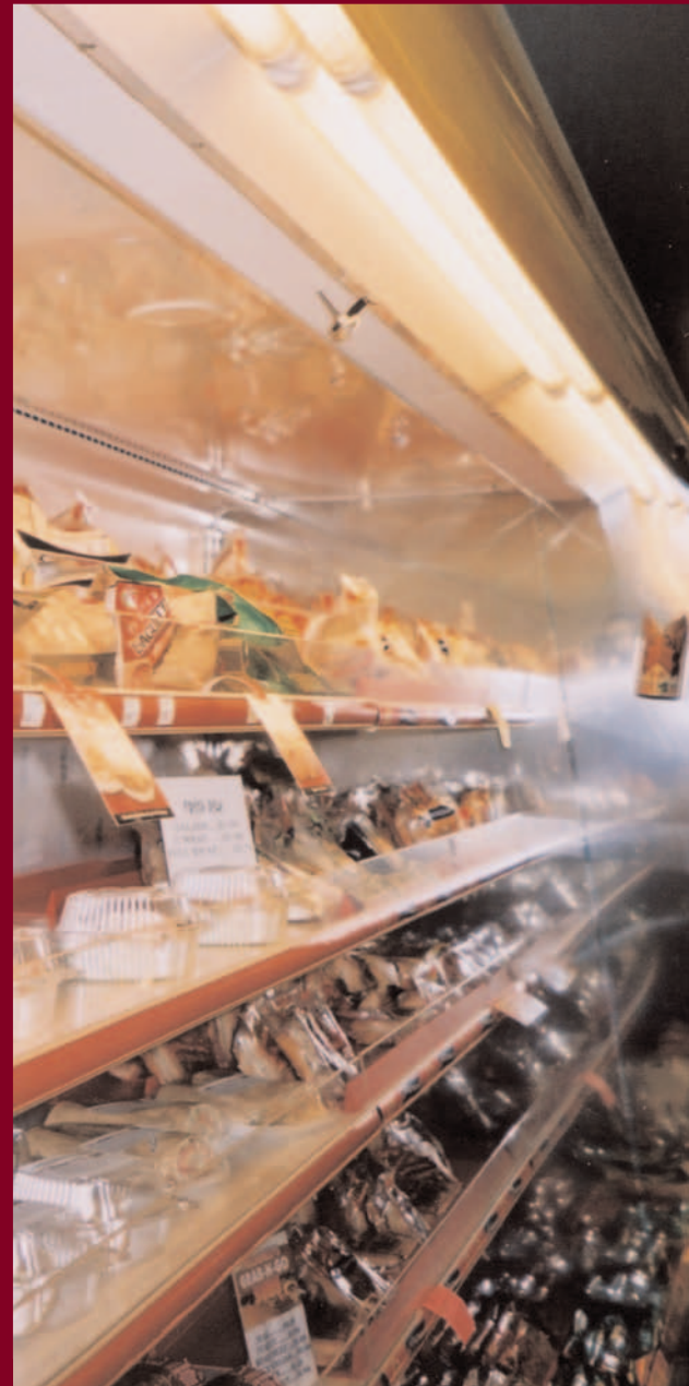
High performance fluorescent lighting in coolers saves money and renders accurate colors for more appealing displays.
