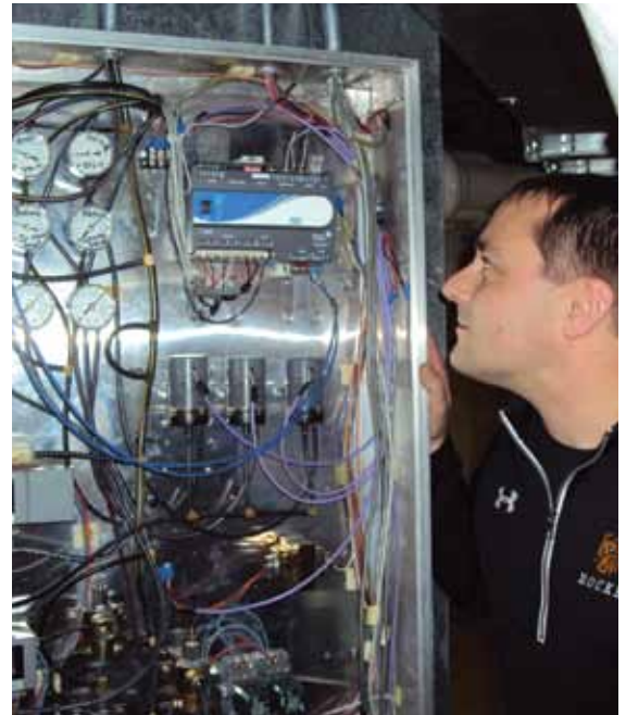
DECC Chief Engineer Wade Abrahamson with heating and cooling controls.
