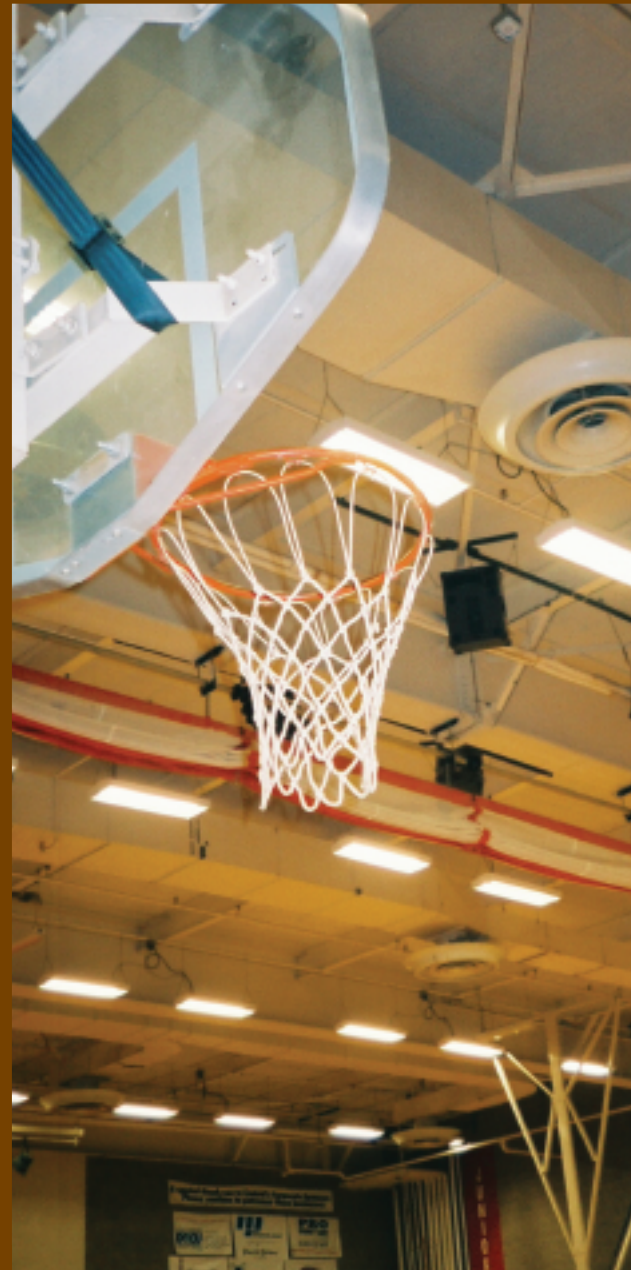
Gymnasium lighting improvements at Duluth Central High School model those tested at Lester Park and are expected to yield substantial energy and cost savings.
