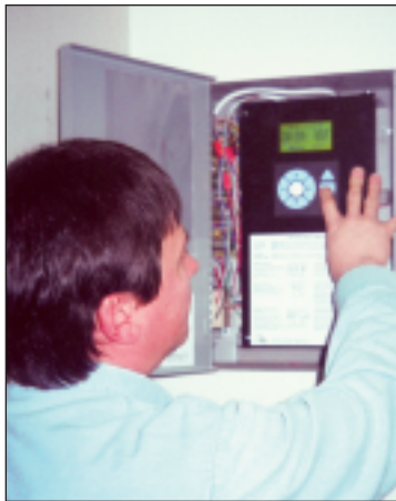
Duluth Schools Master Electrician Gene Salmi programs the gym lights at Lester Park Elementary.
