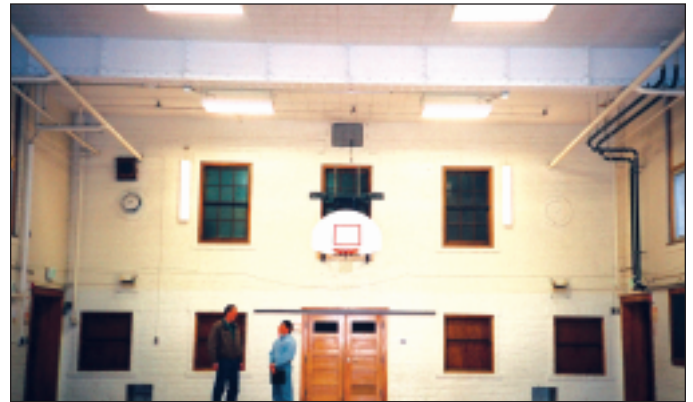
New high-bay fluorescent fixtures and lighting controls cut the electrical costs of lighting the Lester Park gym by 70%, from $524 to $156 per year.
