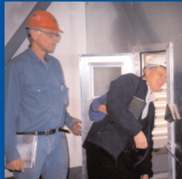
MP energy consultant Gary Olson of Matt Haley & Associates identifies energy-saving technologies and estimates their cost-saving potential for clients. Also shown in bottom photo is foreman Donald Wick, Jamar Co.
