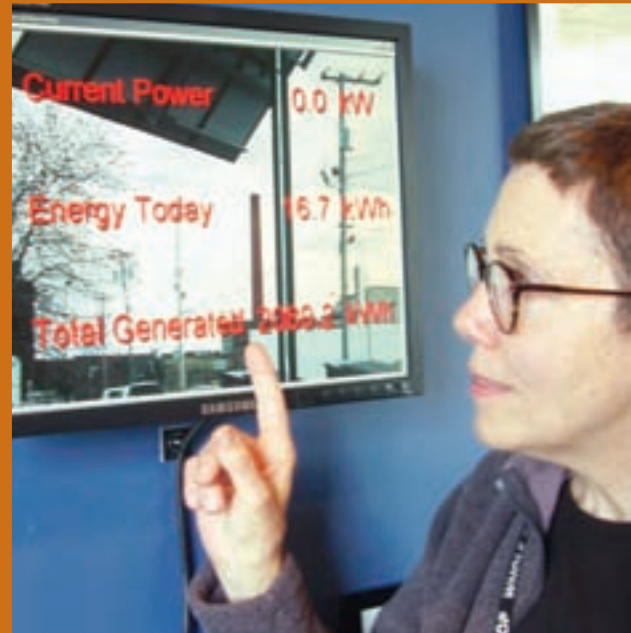
A grid-connected solar photovoltaic system generates a portion of the store's energy. An LED screen inside Whole Foods Co-op displays solar energy data.
