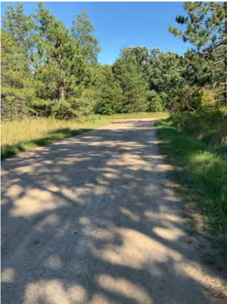
Date: 2024-08-31 Location: 46.3174°, -94.4860° Description: Potholes along the access road
