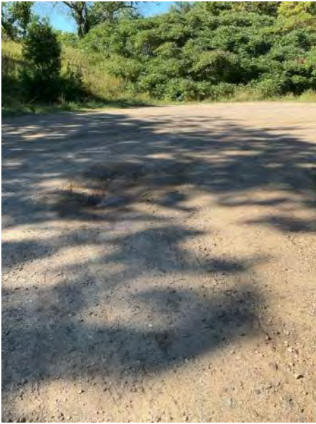
Date: 2024-12-19 Location: 46.3109°, -94.3836° Description: Boat launch parking lot rutting
