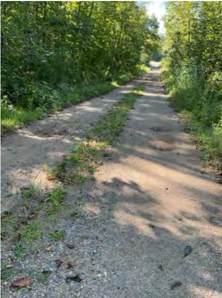
Date: 2024-09-01 Location: 46.3052°, -94.5478° Description: Potholes along the access road
