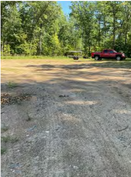
Date: 2024-08-31 Location: 46.3042°, -94.3761° Description: Large ruts and depressions within the parking lot
