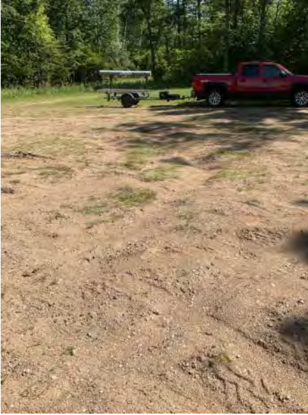
Date: 2024-08-31 Location: 46.3041°, -94.3759° Description: Large ruts and depressions within the parking lot
