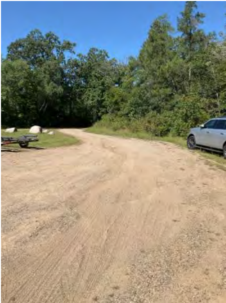
Date: 2024-08-31 Location: 46.3257°, -94.4105° Description: Minor rill erosion
