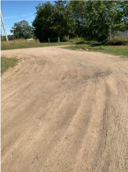
Date: 2024-08-31 Location: 46.3168°, -94.4867° Description: Depression around the parking lot
